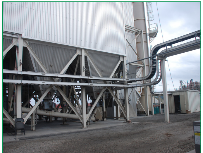
Figure 6. The baggers at the plant collecting the fine ashes and large particles from the gas waste product the process produces.
