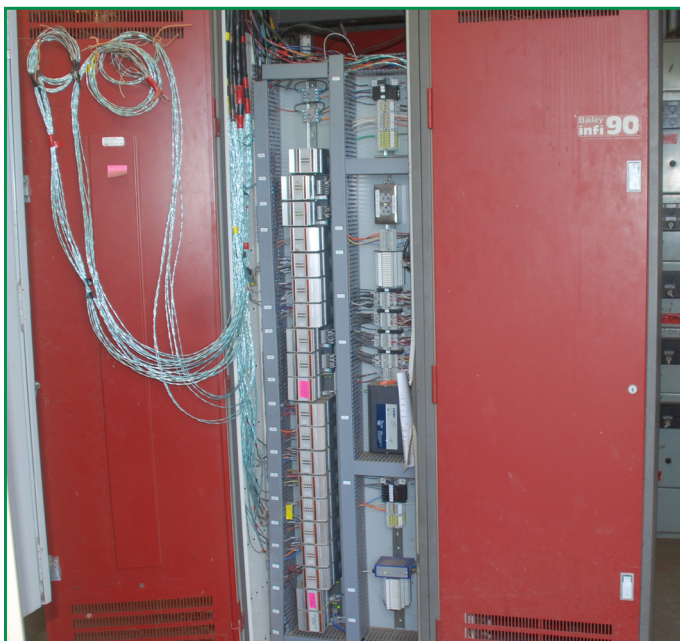
Figure 5. New Ethernet based NCS electronics in the original cabinets at IVRR.
