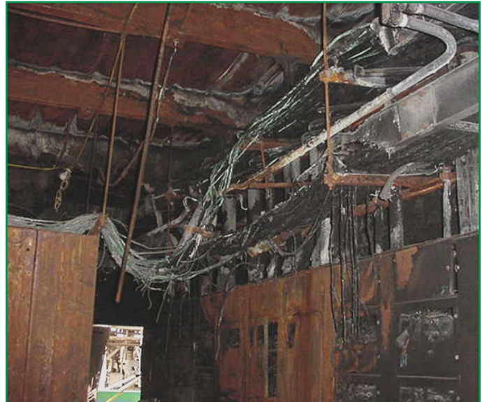
Figure 3. AC Power Panel Room after plasma fireball destruction. Although there is incredible damage to the panel room and control center of IVRR, the rest of the plant is not compromised.
